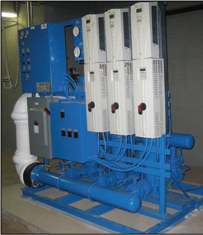
FIGURE 1. The VFD-driven triplex house booster pump set.
