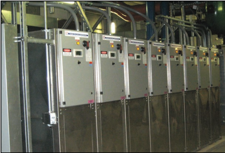
FIGURE 3. The modular chiller set, supplied by Tandem Chillers, Inc.
