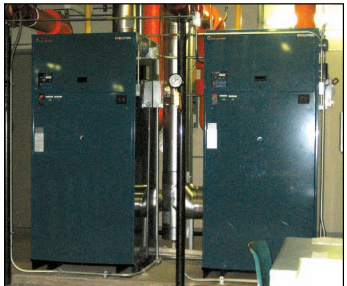
FIGURE 2. Duplex gas boiler set.
